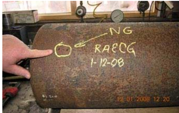
Holes in the main reservoir
