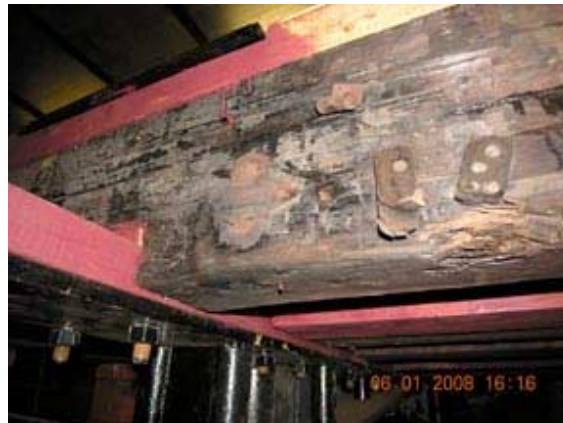
Sill 6 showing charred area of wiring fire in motor no. 4 leads,
