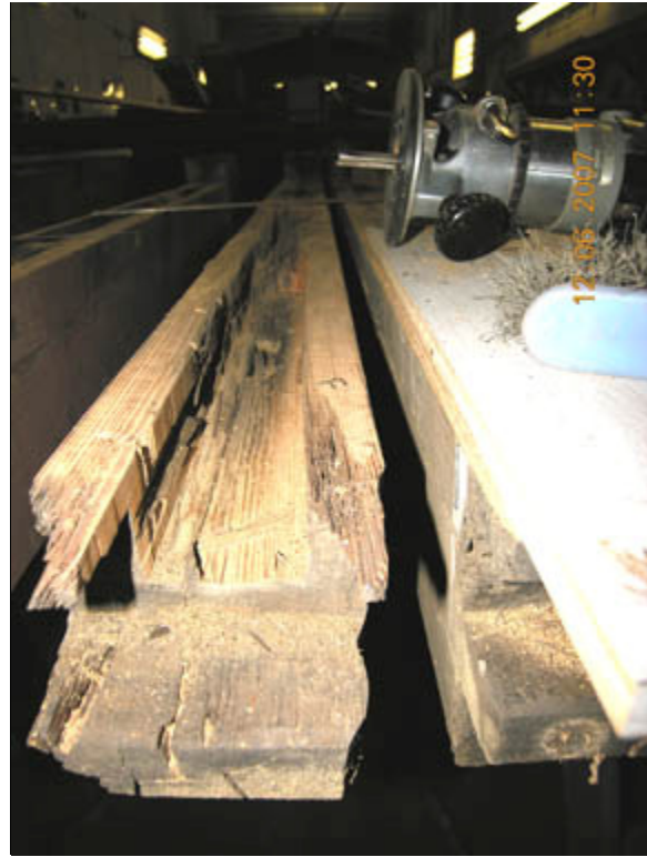
Sill 5 with rotted area routed out
