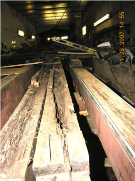
Sills 5 & 4 showing deteriorated areas
