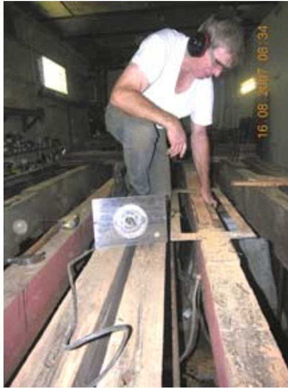
Hollowing out deteriorated sill
