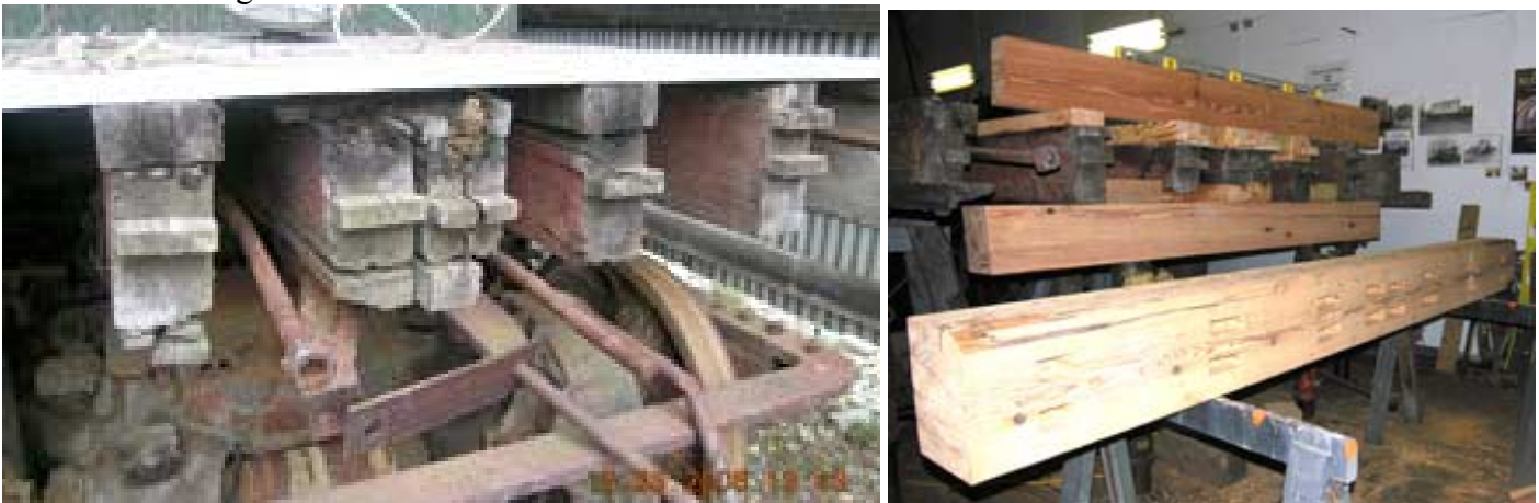
Before and after showing the tenons on the ends of the long sills and the new end sill ready to fit.
